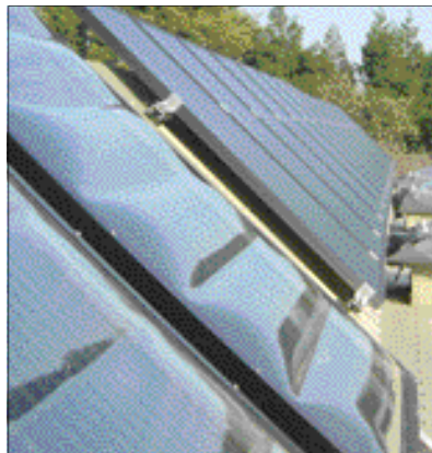
The Earthship Solar Panels
