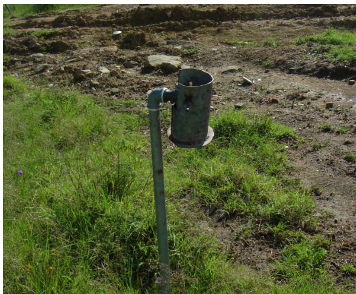
Picture 3: A closed standpipe in a yard in Ha Thetsane
