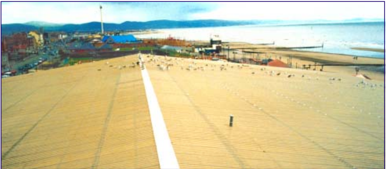
FILON SupasaFe Gold Tint for a Complete Re-roof at Rhyl Suncentre (replacing polycarbonate)
