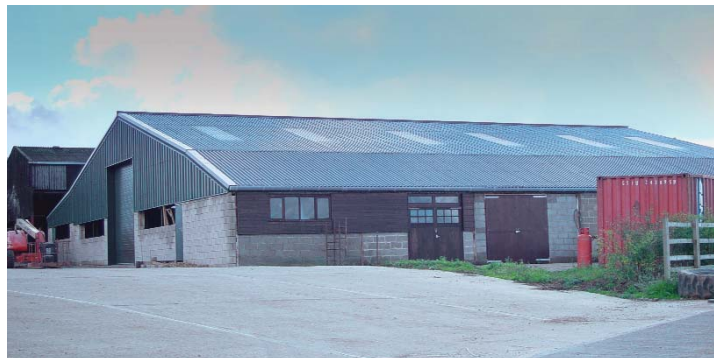
Former cowshed at Shack's Barn Farm, Silverstone. FILON over-roofing allowed the building to be upgraded for commercial use.
