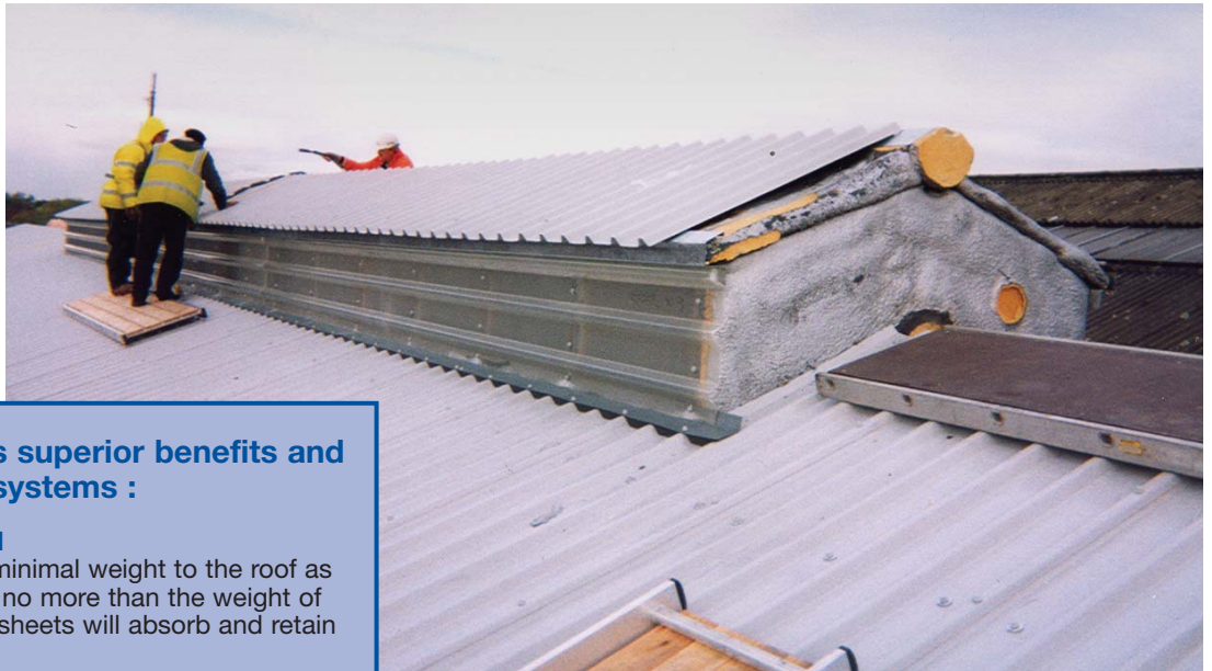
This roof in Darlington, had previously been sprayed with urethane foam in an attempt to cure water ingress. The foam had reacted to the asbestos cement, resulting in increased water ingress. FILON over-roofing solved the problem.
