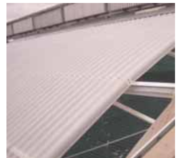
FILON rooflights were specifically designed for the curved roof.
