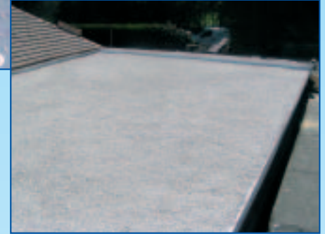
The finished roof – excellent aesthetics and effective performance with a 25 year guarantee
