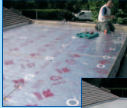
Before the GRP TecnaFlex sheets are applied, the insulation layer and MAP (Mobile Anchor Plate) fixings are visible.
