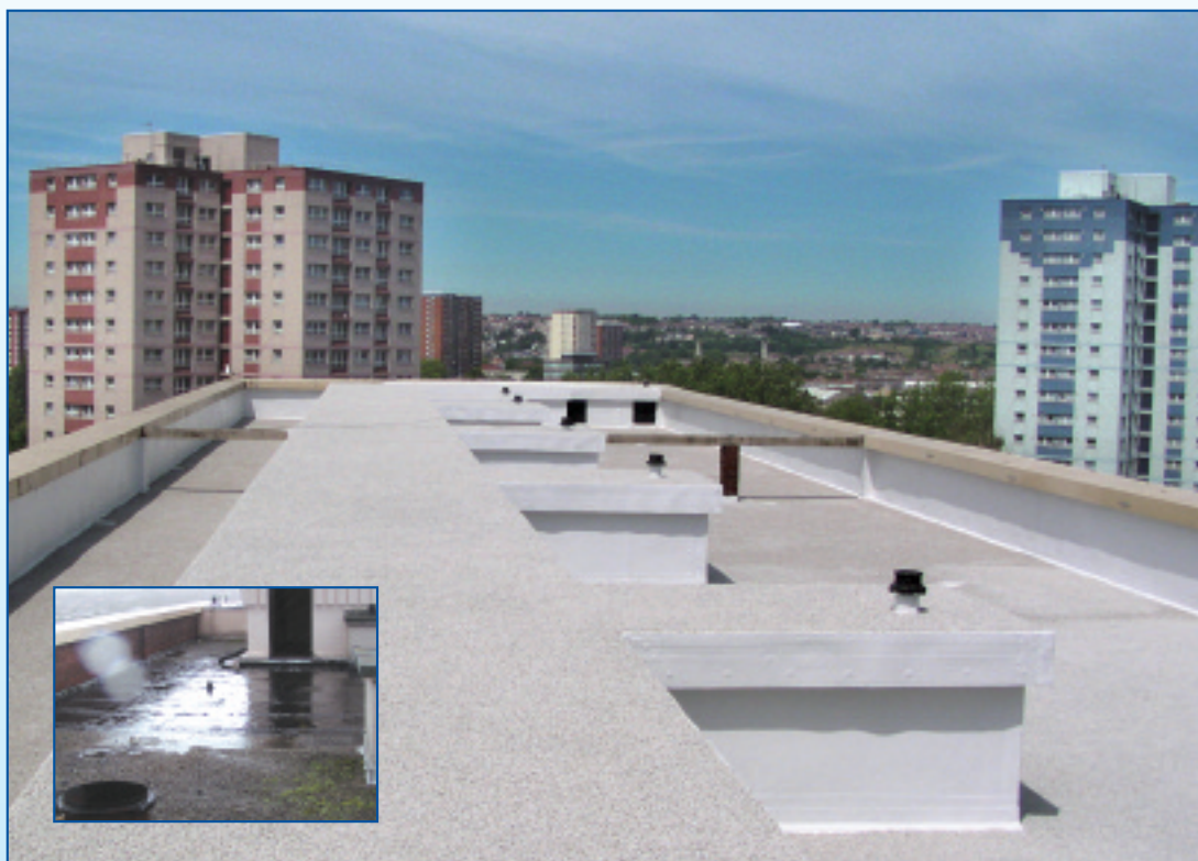
The roof at Ecclestone House, Bristol, before and after installation of the new Tecnaflex system
