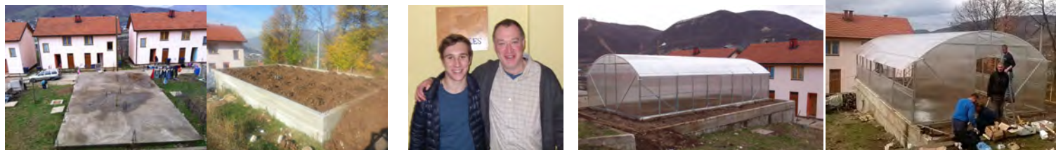
Above Left to Right: the first base is ready for the greenhouse to be installed then the concrete base is laid and filled with earth.
