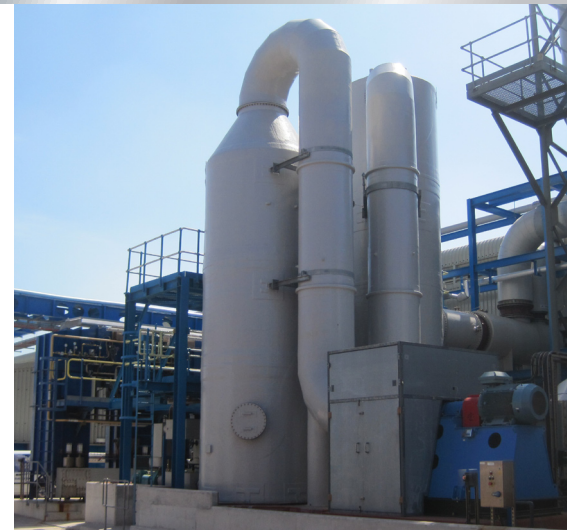
Flue gas treatment for manufacture of alumina based fibre, UK
