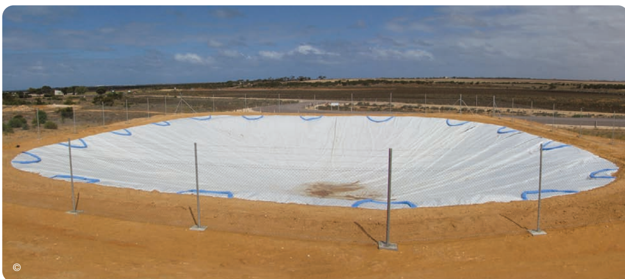
VapourGuard installation by Fabtech SA Pty Ltd in Arno Bay, South Australia (1,800m 2 )
