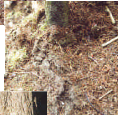
Ground heave adjacent to tree.
